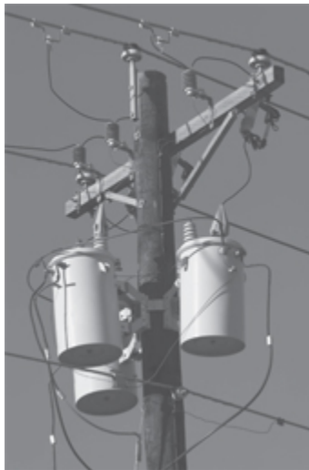
Three transformers on a neighborhood power distribution line.
